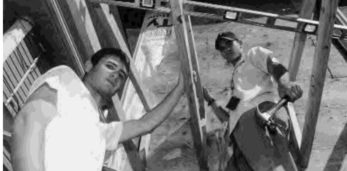
Nail by nail, Seton Hall students donate their time to Habit for Humanity in Newark, as part of the volunteer corps that builds homes for low-income families.
